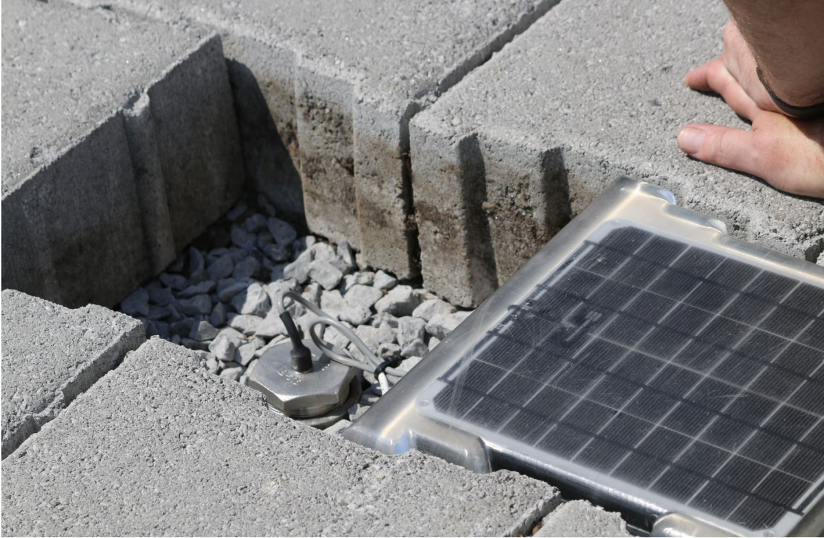
Figure 5. Solar-powered INFIL-Tracker PaveDrain block (right) connected to underground sensor (left) located beneath adjacent sensor cover block.
